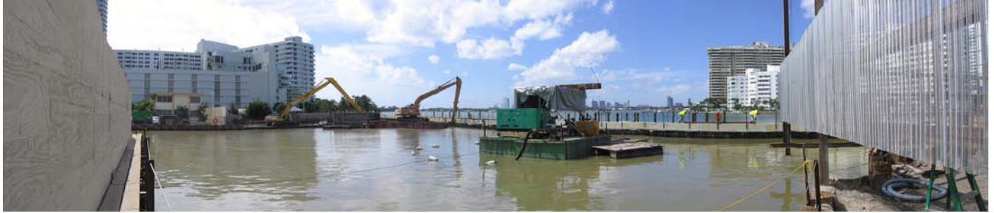
Wide angle view of the Capri Residence site being prepared to receive the Tremie slab
