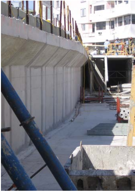
A view from inside the "bathtub" showing the retaining wall and slab
